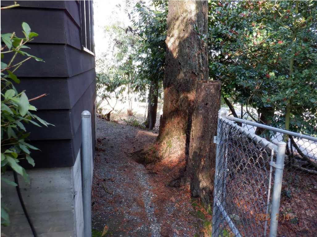
Tree #13 located close to existing structure
